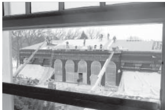
Construction photo of the McEssy Theological Resource Center at the University of Saint Mary of the Lake/Mundelein Seminary, home of the Liturgical Institute.
